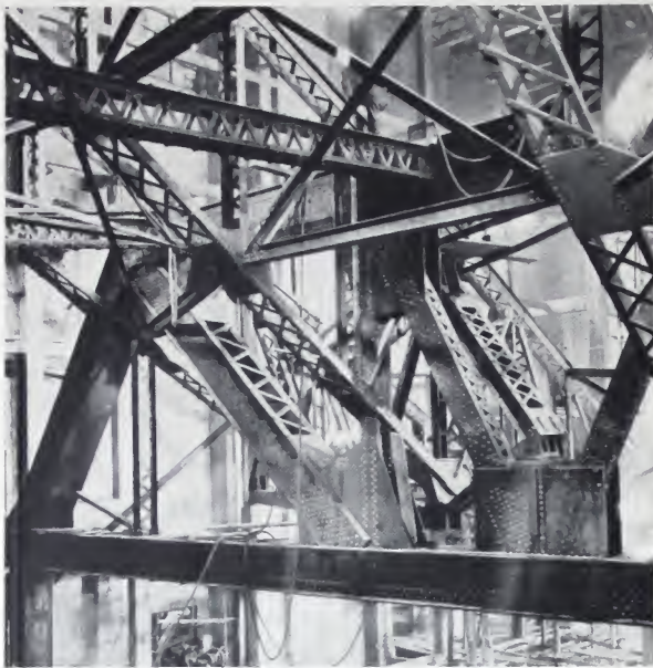
MAIN BALCONY TRUSS SHOWING PIN COLUMN CONNECTION AND PIN CONNECTION OF JACK TRUSS TO STEEL CASTING ON MAIN TRUSS. ABOUT 30% OF HOLES IN CONNECTIONS WERE BOLTED TIGHT BEFORE ONE INCH TAPERED RIVETS WERE DRIVEN UNDER 120-LB. PRESSURE
